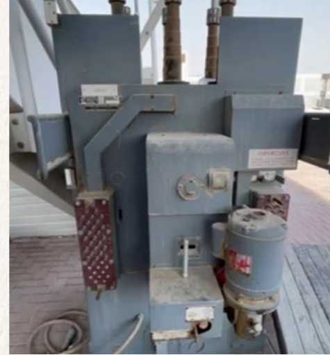
33kv South Wales Circuit Breaker
